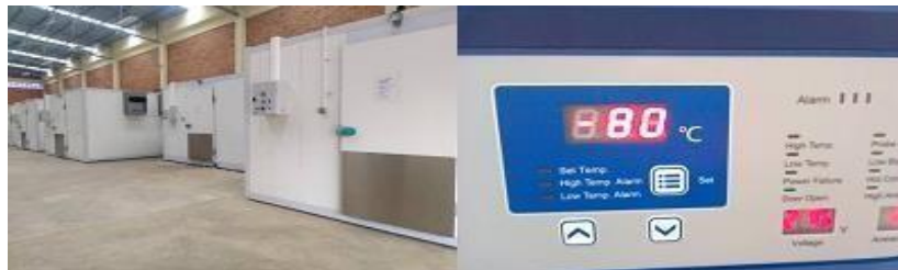
Figure2. Purchased equipment for storage of vaccines
