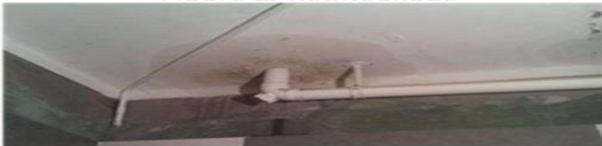
Figure 3: Kitchen and toilet leakage
