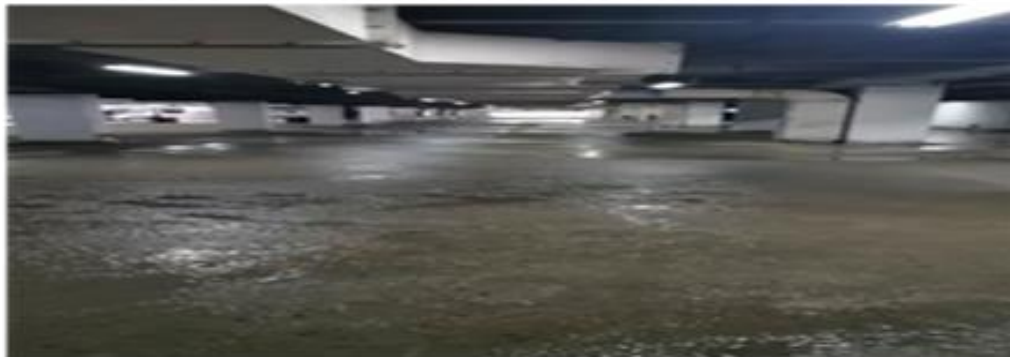
Figure 4: Basement and underground parking leakage
